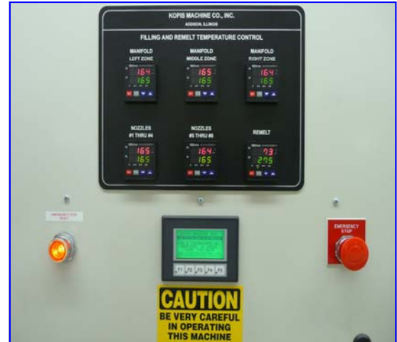
Operator HMI and Heater Control Panel
