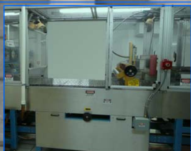
Operator Access Area Re-melt Unit on Right
